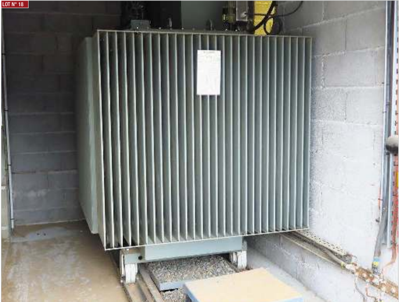
► Transformateur triphasé CAHORS (2015), 2500 Kwa, tension primaire 20 000 V, tension secondaire 410 V ► CAHORS three-phase transformer (2015), 2500 kWA, primary voltage 20,000 V, secondary voltage 410 V
